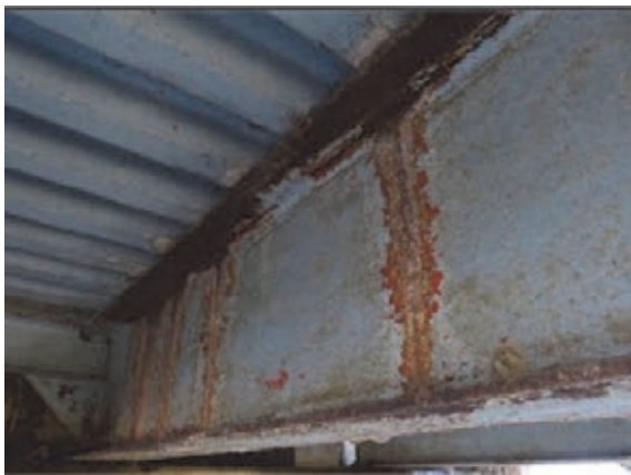
(a) 腐食①
